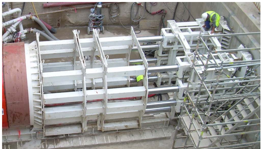
A 1600 tonne Compact Jacking Rig is seen installing a 3020mm O.D. machine in Barcelona.
