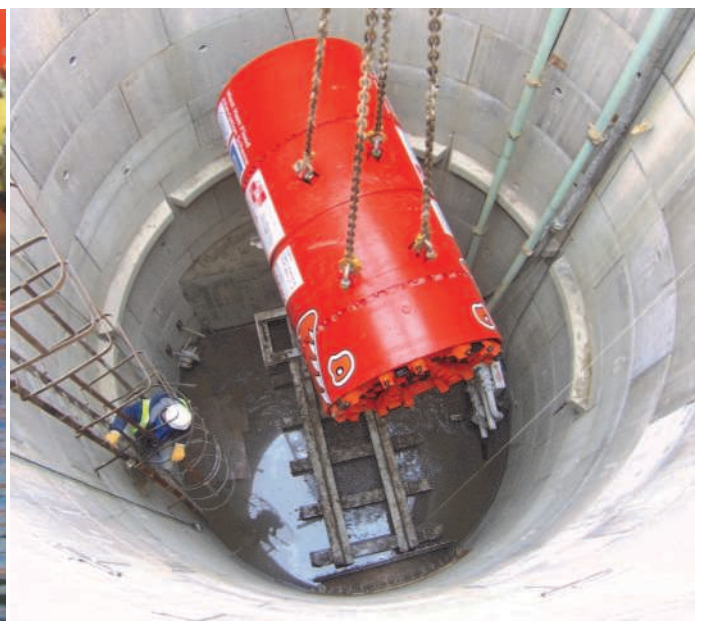
The machine is lowered into the jacking shaft at the beginning of the West Ham (IV) project in London
