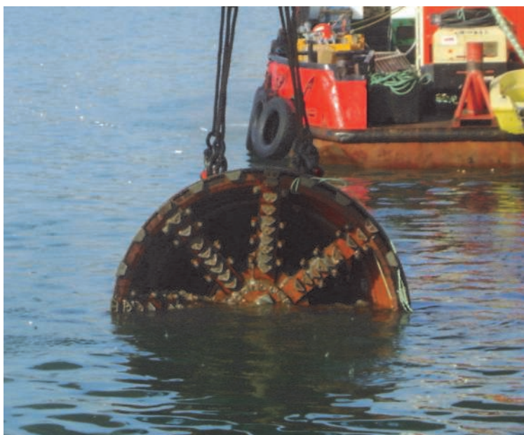
The TBM is lifted out of the water at Barcelona after completion of a sea outfall pipeline
